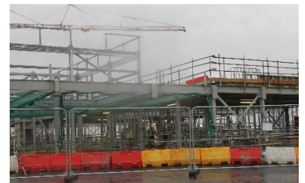
The Springwell Leeds, North site with the crane waiting to lift the final piece of the structure.
